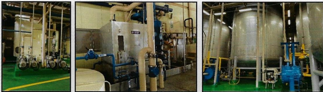
<Fig. 9> Test configuration scenes (the cooling water tank and pump, chiller, ferment tanks)
